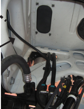
Place corner guards to protect wiring
